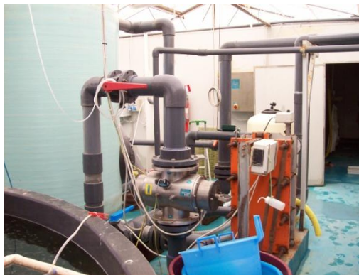
Figure 3: An HydroFLOW A100 unit installed before the water is transferred to the main fish tanks.
