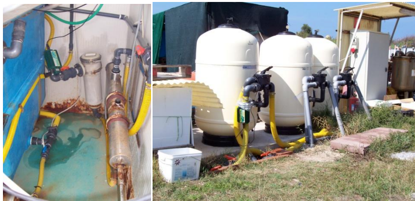
Figure 6: External water storage tanks also had their UV protection replaced with HydroFLOW.
