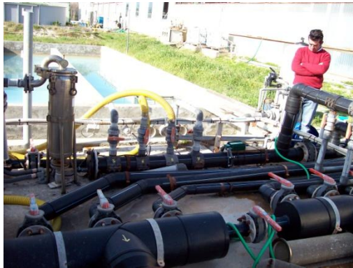
Figure 2: An HydroFLOW unit installed on the incoming water to the whole plant.
